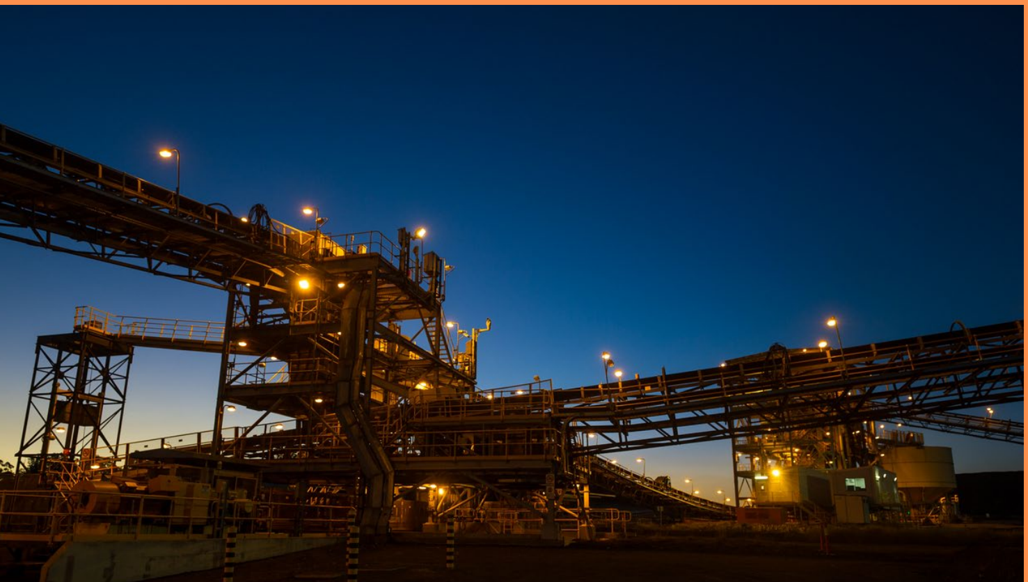
Mining processing plant with illuminated conveyor belts and steel structures at dawn.
